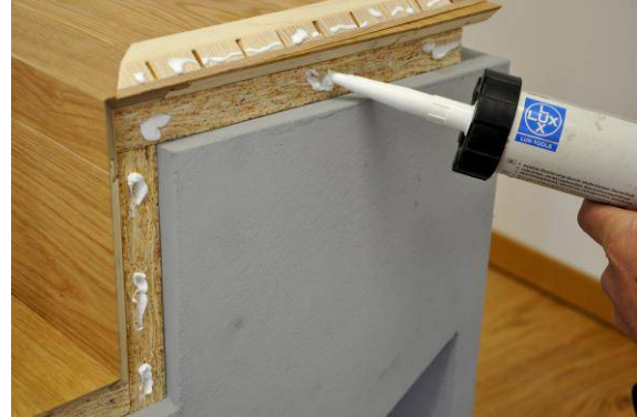
Once the precision fit of the panel has been checked and the panel re-cut if necessary, it is glued at the mitre joint using a fast-drying PVAC adhesive and glued additionally at the outer edge of the shim with the synthetic resin adhesive.
