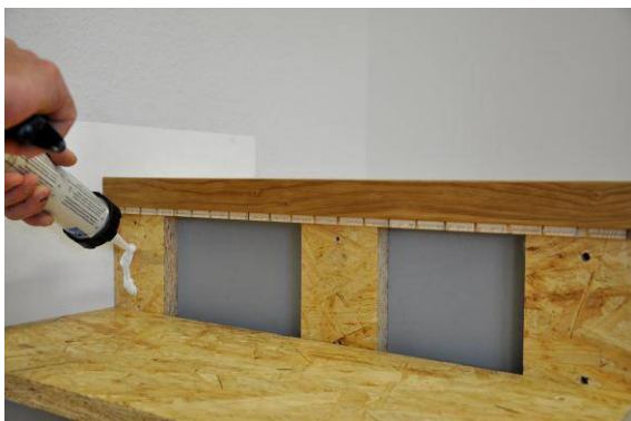
A synthetic resin adhesive is applied to the front of the riser shim to glue the riser.
