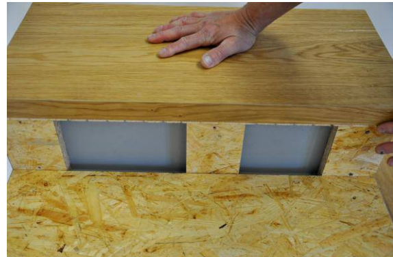
Insert the individual pieces in succession into the glue layer and ensure proper coverage with the glue.
