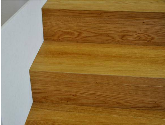
All other steps and risers are adjusted and glued in succession as described above. The precision fit to the wall is also important to ensure here.
